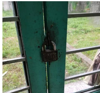
Figure 3: Locked Exit Door
