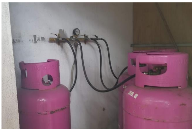
Figure 10: Gas Cylinder on Left Not Connected to Emergency Shut-Off
