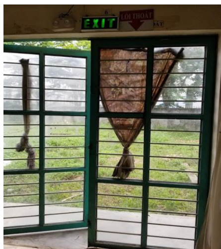
Figure 2: Exit Door ‘Pinned’ Partially Open
