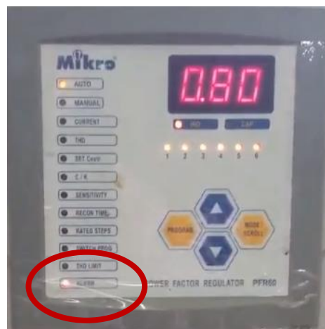
Figure 28: Electrical Panel with "ALARM" Warning Lit
