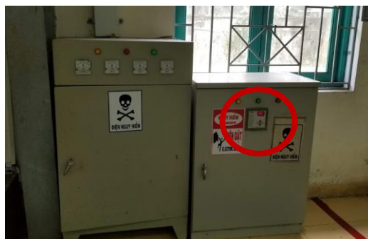
Figure 27: Main Electrical Panels
