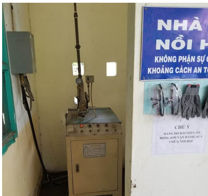
Figure 14: Steam Compressor with Only Safety Glasses and Gloves Provided for PPE
