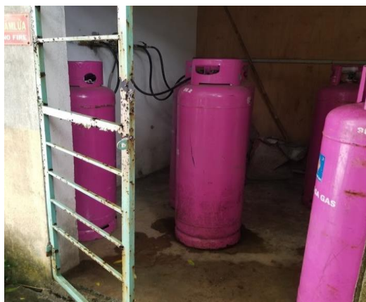
Figure 9: Unsecured Gas Cylinders
