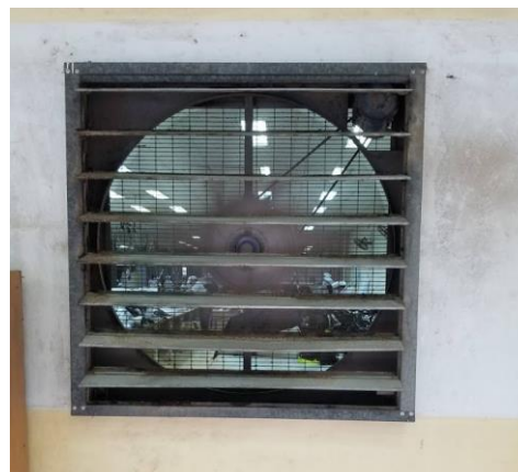
Figure 16: Unguarded Fan Blades inside Dampers
