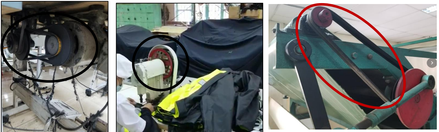
Figures 20-22: Lack of Guarding on Belt-Driven Machines
